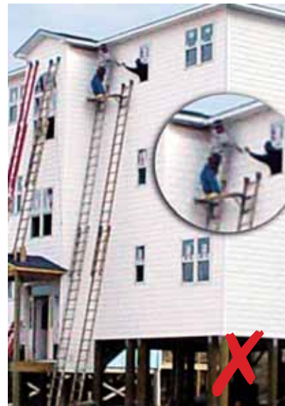
An accident waiting to happen.
